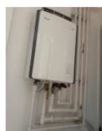
Gas water heater
